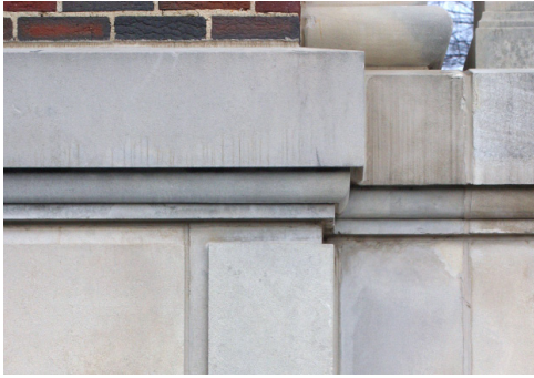
Above: Water table is sloped to shed water and protect stonework below.
