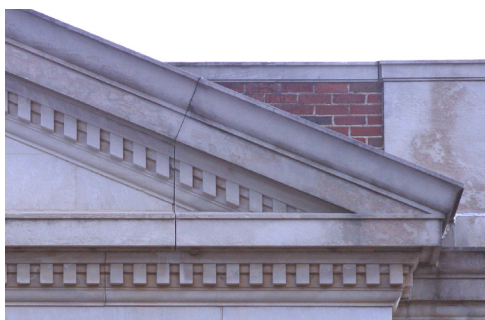
A product of the pitched roof design is the tympanum or triangular pediment at the gable end. Where it occurs, this element is part of the crown. The tympanum is surrounded by projections of the cornice profiles.
